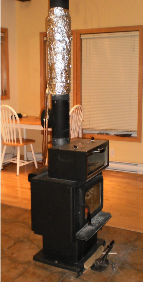
Photo-1 Un-shrouded stove-pipe heat-exchanger
